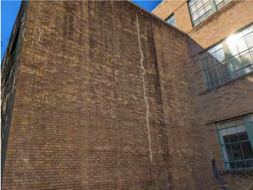
Photograph 5: Evidence of cracking and deterioration of exterior wall
