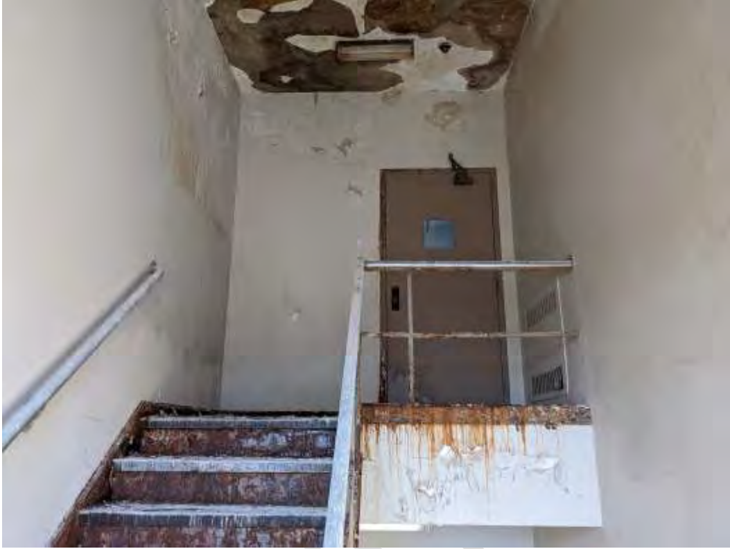
Photograph 13: Evidence of water damage (Building 3)
