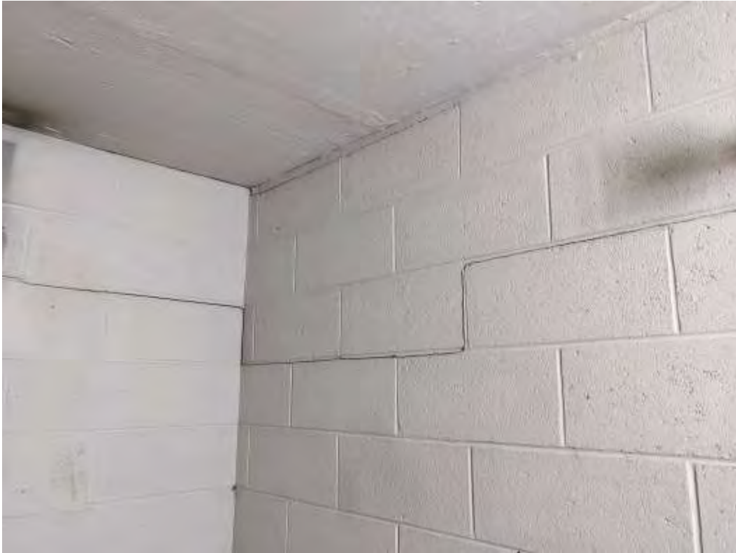
Photograph 7: Evidence of cracking and deterioration of stairwell
