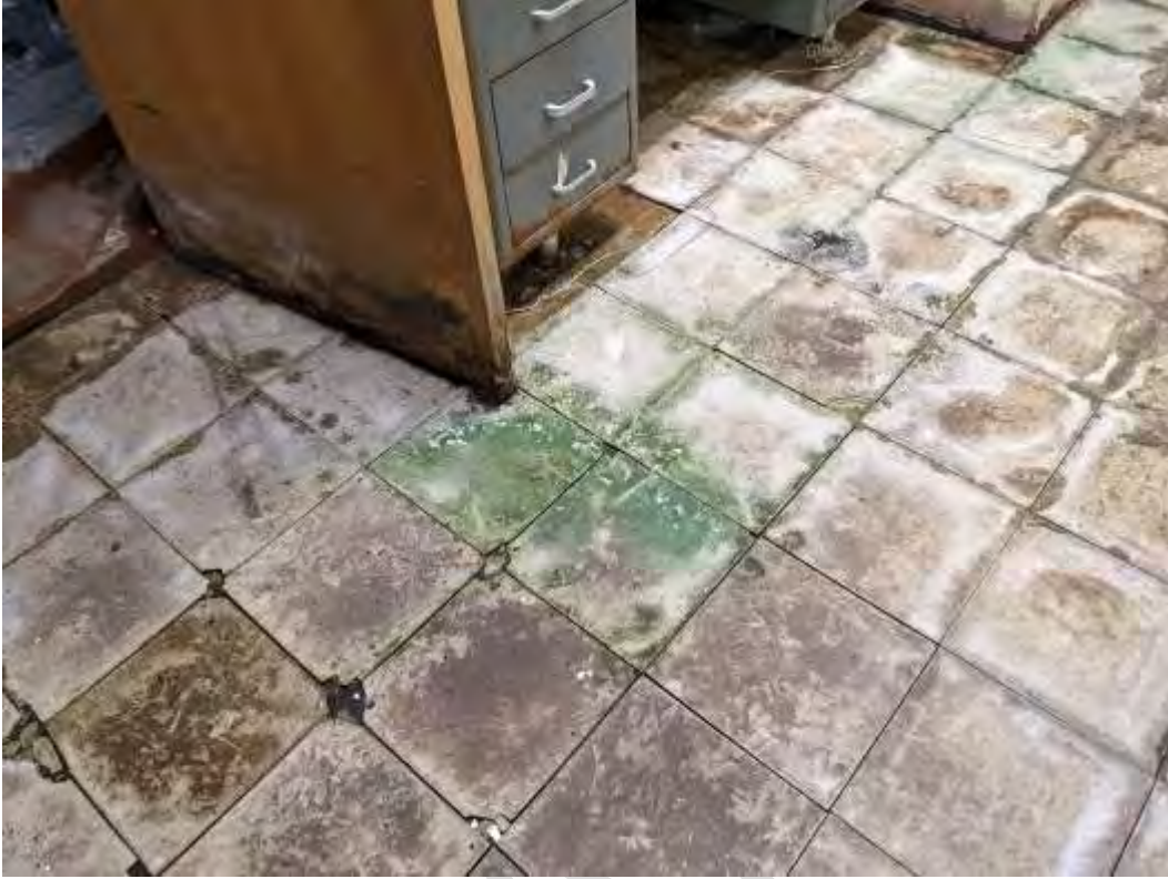
Photograph 11: Evidence of water damage (Building 4)
