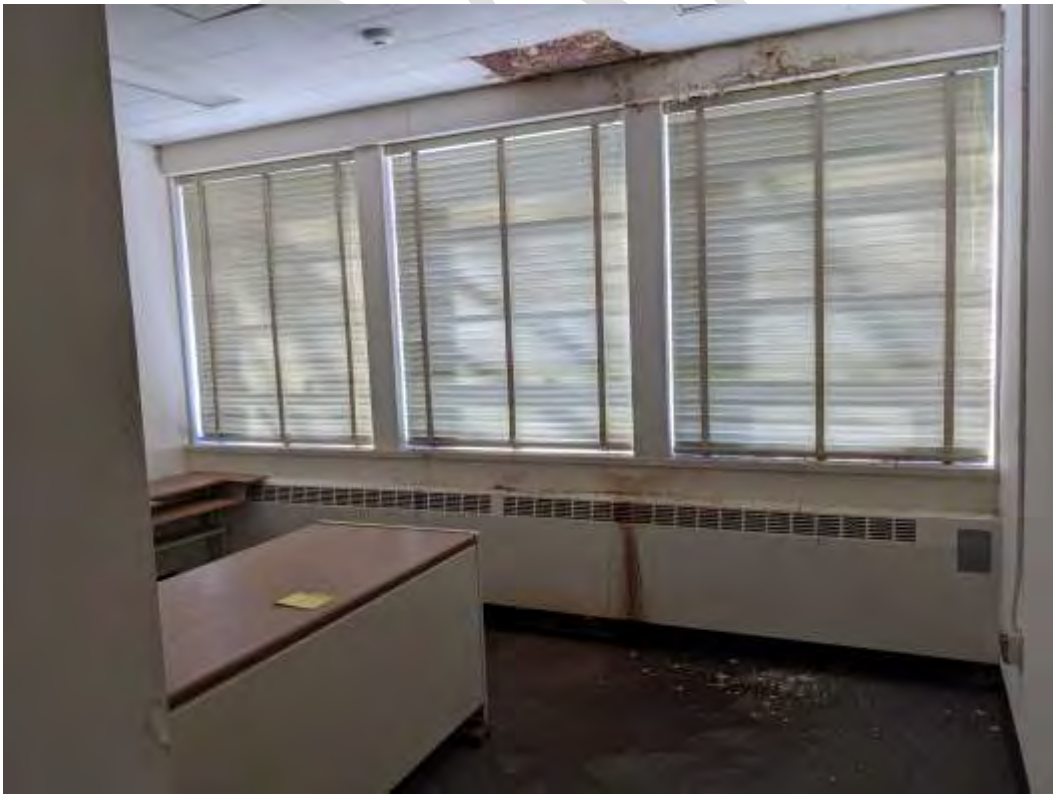
Photograph 15: Evidence of water damage (Building 3)
