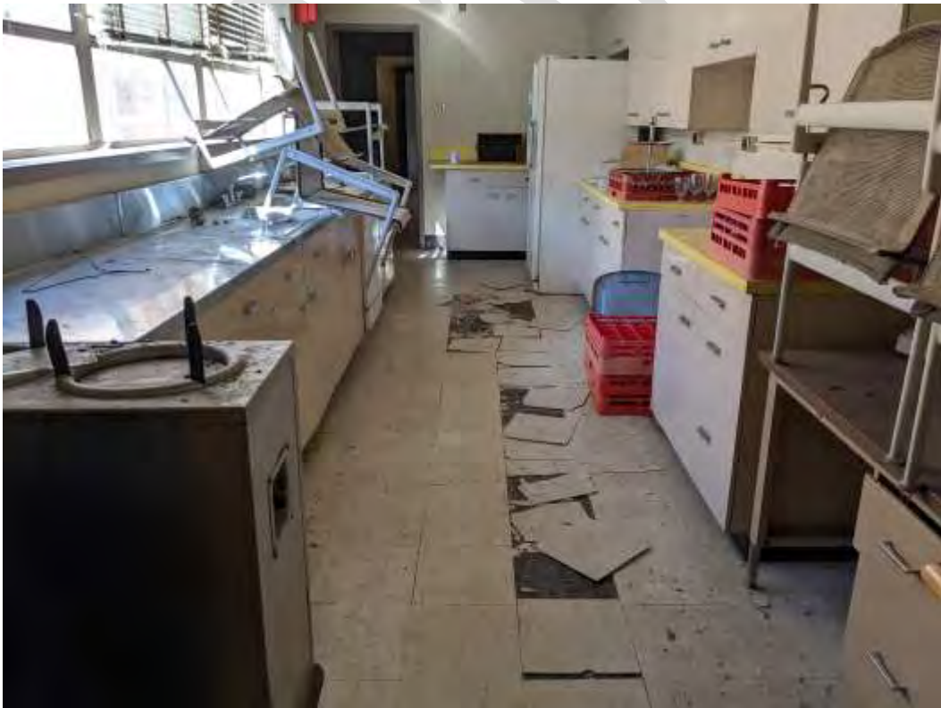
Photograph 17: Evidence of water damage
