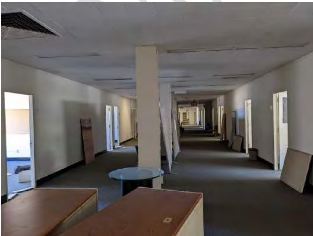
Photograph 27: Evidence of vacant space (Building 3)
