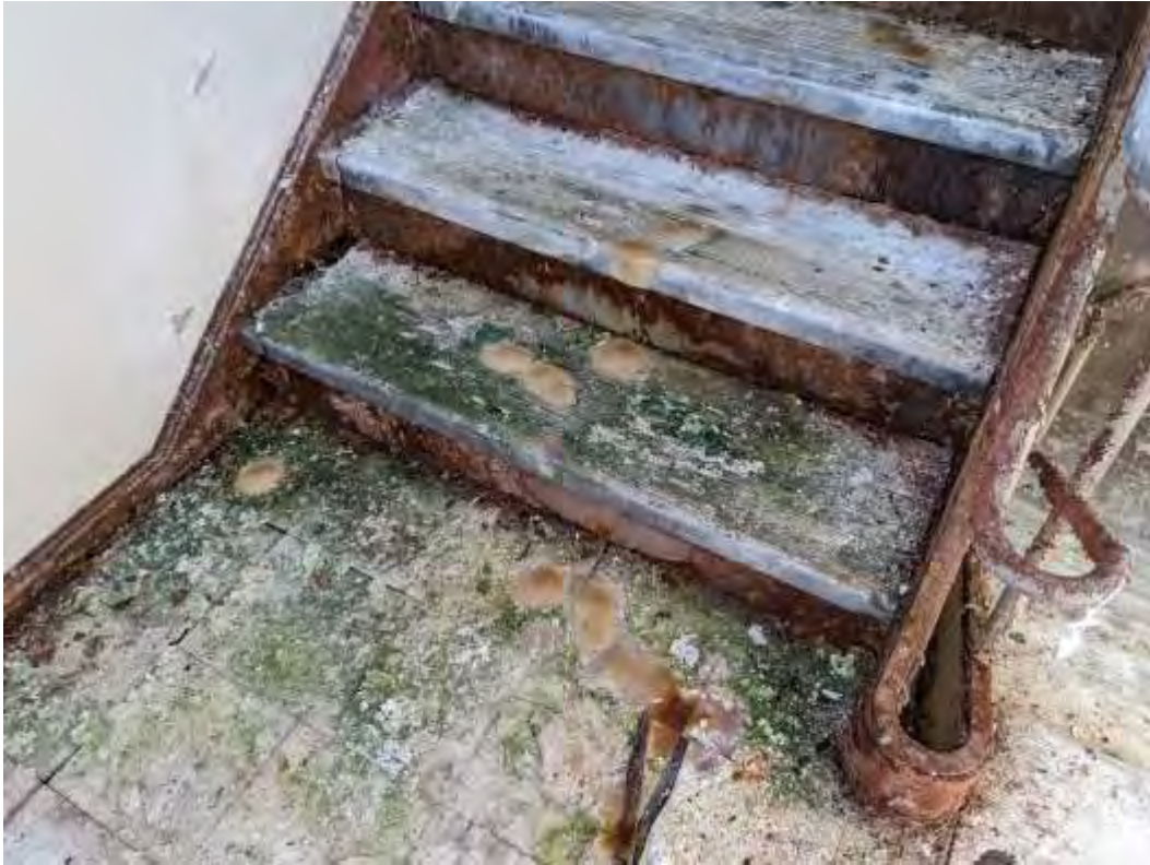
Photograph 14: Evidence of water damage and mold (Building 3)
