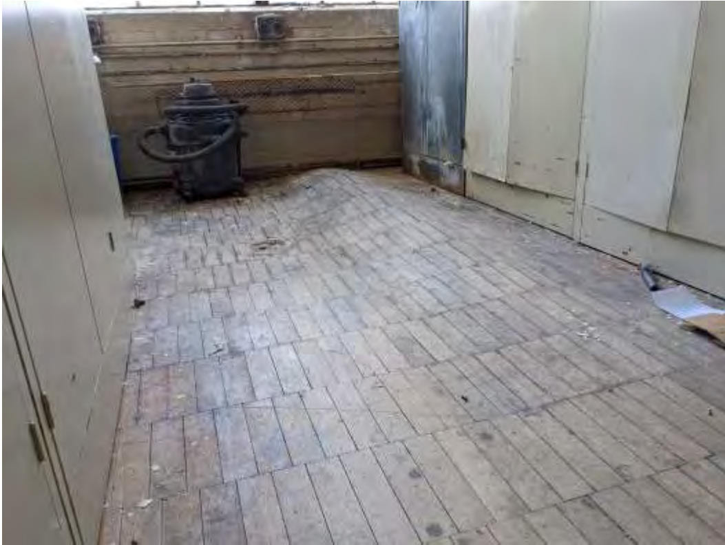
Photograph 16: Evidence of water damage and warped floorboards
