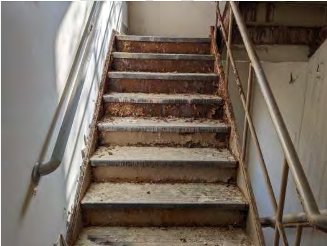
Photograph 12: Evidence of water damage (Building 3)
