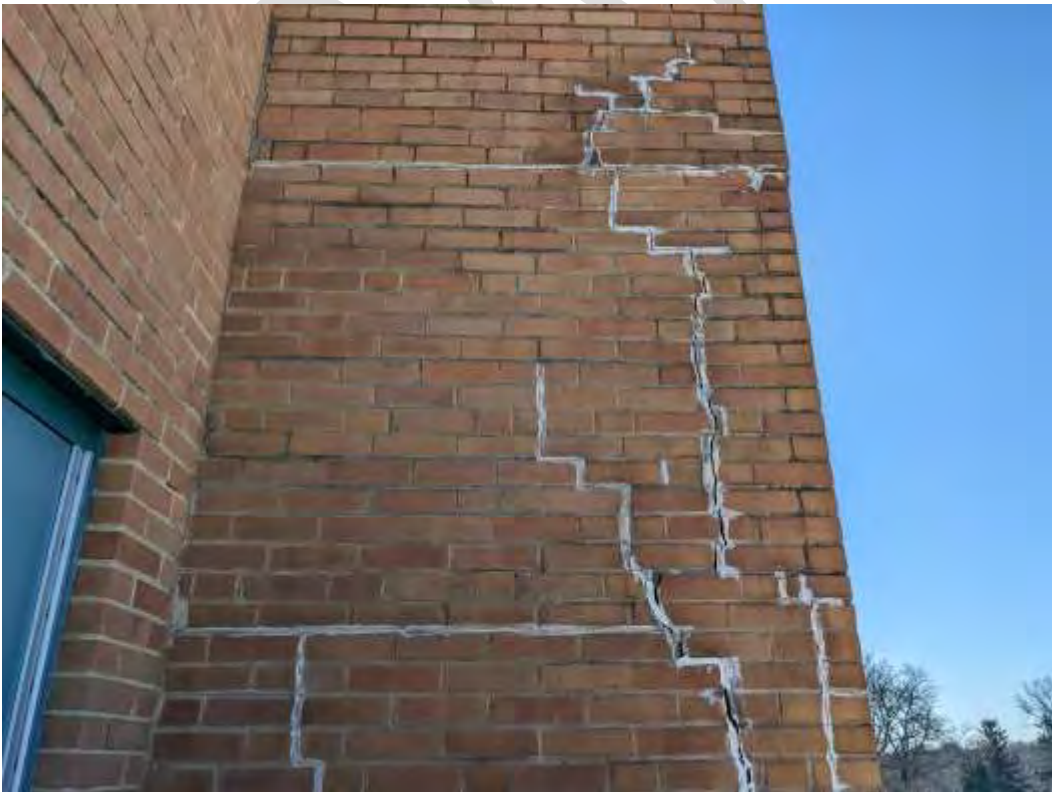
Photograph 4: Evidence of cracking and deterioration of exterior wall
